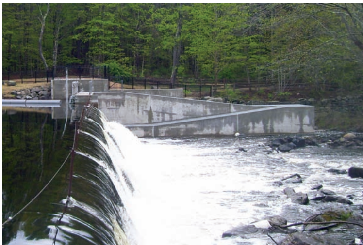
Newly installed Wiswall Fish Ladder on the Lamprey River, Durham, NH. Photo by D. Cedarholm
